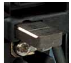
Visual inspection of carbon brushes is rather simple due to the markings as applied.
