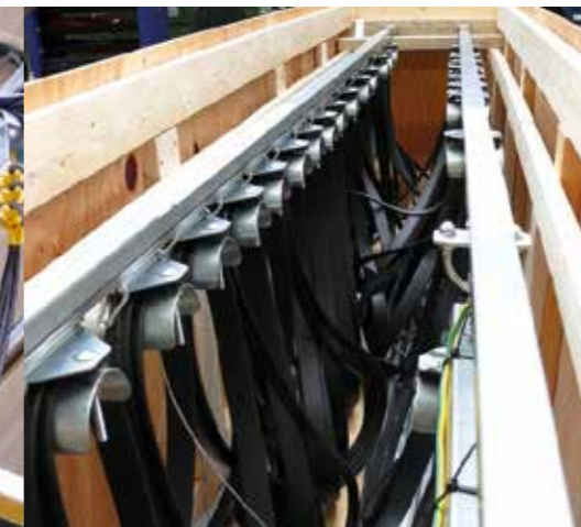
Ready to use hoist power supply
